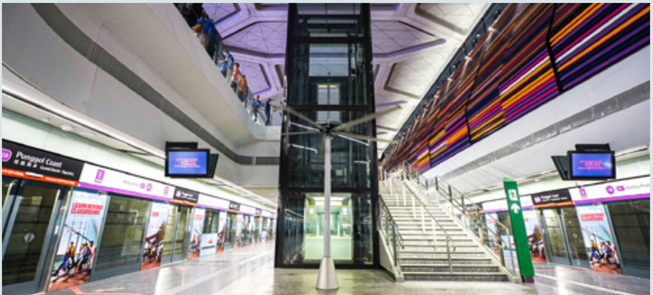
Hybrid fans at the platform are used in conjunction with the Punggol Digital District's District Cooling System to keep the station feeling cool while utilising energy efficiently.
